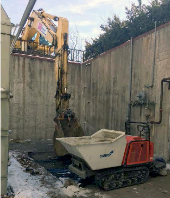
The excavator bucket was used to transfer the waste from the basement walkout up to the dump truck in the parking lot.
