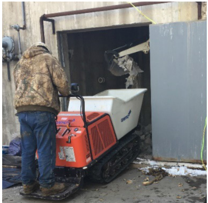
The vault was 10’x12’, so it was tight quarters, even for a mini-excavator.
