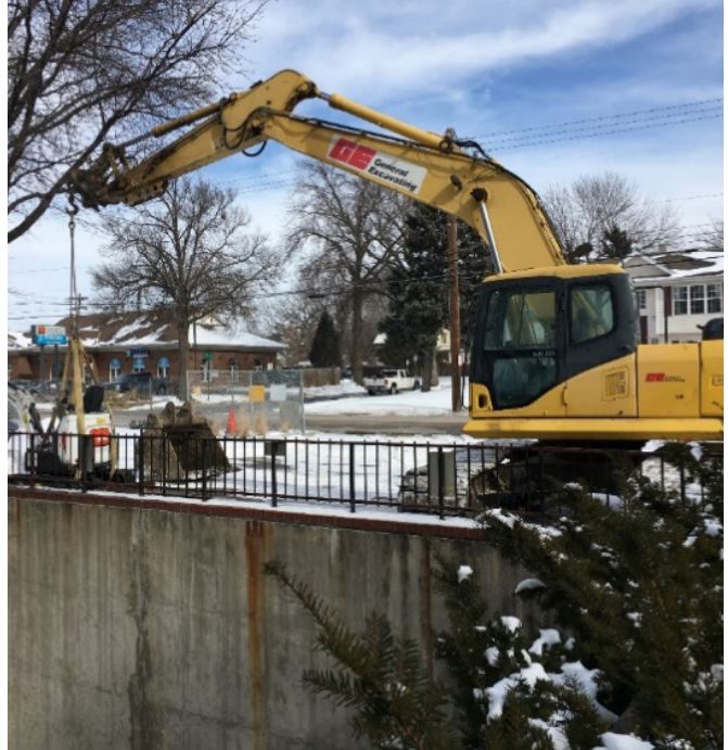
The vault entrance was located 14’ below-grade with access from the basement walkout where the HVAC heat exchange units were located. All the equipment that used was lowered into the area with the excavator.
